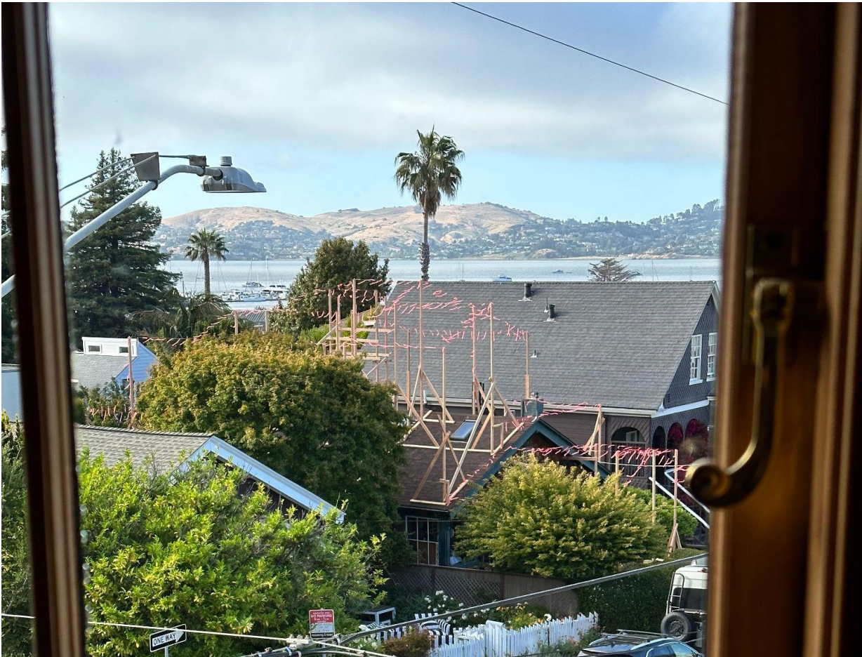
Image 1b: View from 19 Bonita of the Schoonmaker Point Marina showing no blockage with story poles
